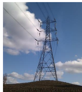
Electricity power line
